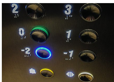
Control buttons in an elevator (lift).
